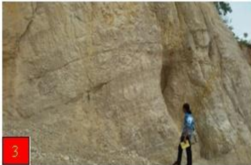
Figure 3: Medium to thick bedded, light grey to grey, highly brecciated and well jointed dolomite and dolomitic limestone of the lower part of Maymyo Formation (N 22° 39' 24" and E 97° 28' 56")
